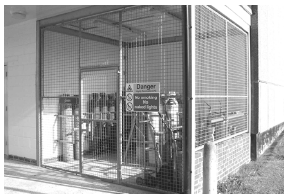
Figure 4: Gas store area
